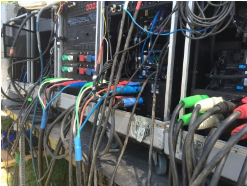
Amp Racks from Monitor World, using an SC48 Console
